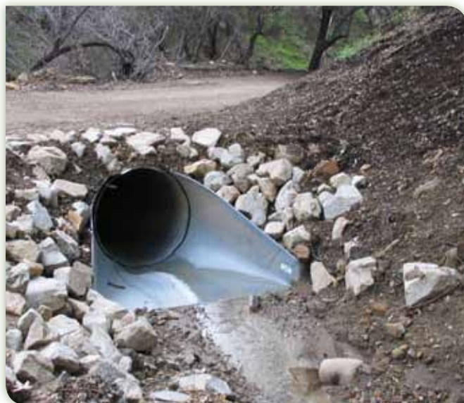
Figure 5. A new, larger culvert and inlet armoring installed after the 2003 Piru Fire in southern California.
