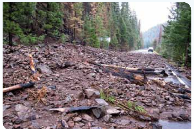
Figure 1. A debris flow blocks the highway following intense rainfall near the 2011 Wallow Fire in eastern Arizona.
