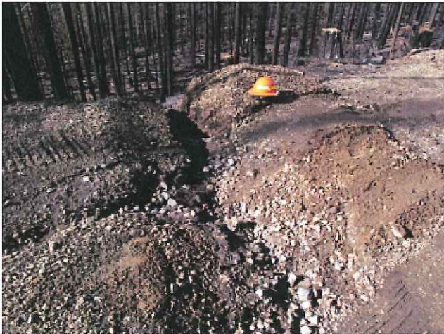
Photo 4. Erosion at waterbar on 8040500 road at MP ~1.1 after receiving moderate rainfall.
