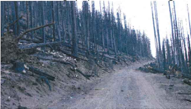
Photo 2. Looking up up 8040500 road in high burn area at MP 1.0 after receiving moderate rainfall.
