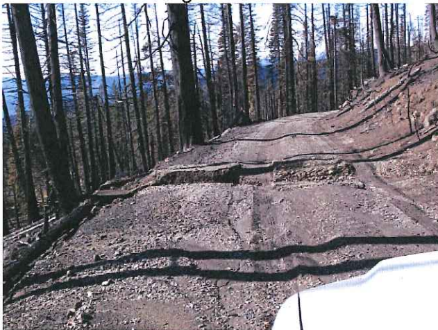
Photo 5. MP Looking down 8040500 road at MP 2.7 after receiving moderate rainfall.
