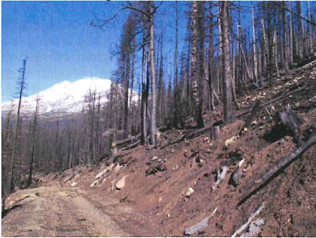
Photo 3. Looking down 8040500 road at MP 1.1 after receiving moderate rainfall.
