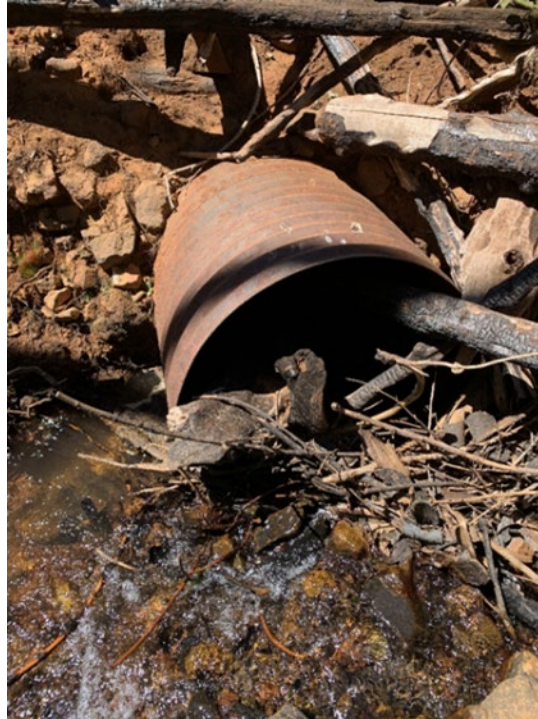
Figure 4. A culvert partially blocked by burned wood and debris in the 2020 North Complex Fire in Butte County, California. In this picture, the road is acting as a partial barrier and a sink for runoff, sediment, and debris.
