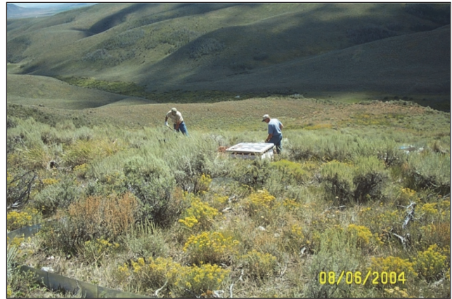
Figure 4. Installation of an unburned plot. Note the upper plot border in the lower left corner and the cover over the tipping bucket installation at the bottom of the plot. The sagebrush canopy is the light green shrub, and the yellow flowering shrub is rabbitbrush ( Ericameria nauseosa ) on the Red Mountain burn erosion study (photo by I. S. Miller).
