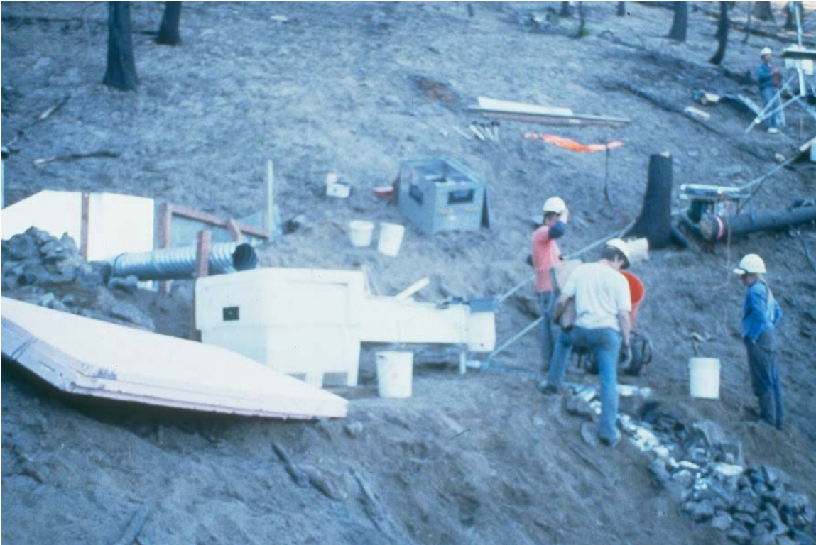
Figure 9. Installing a weir and sediment collector on a site following a wildfire in the Wenatchee National Forest, Washington.
