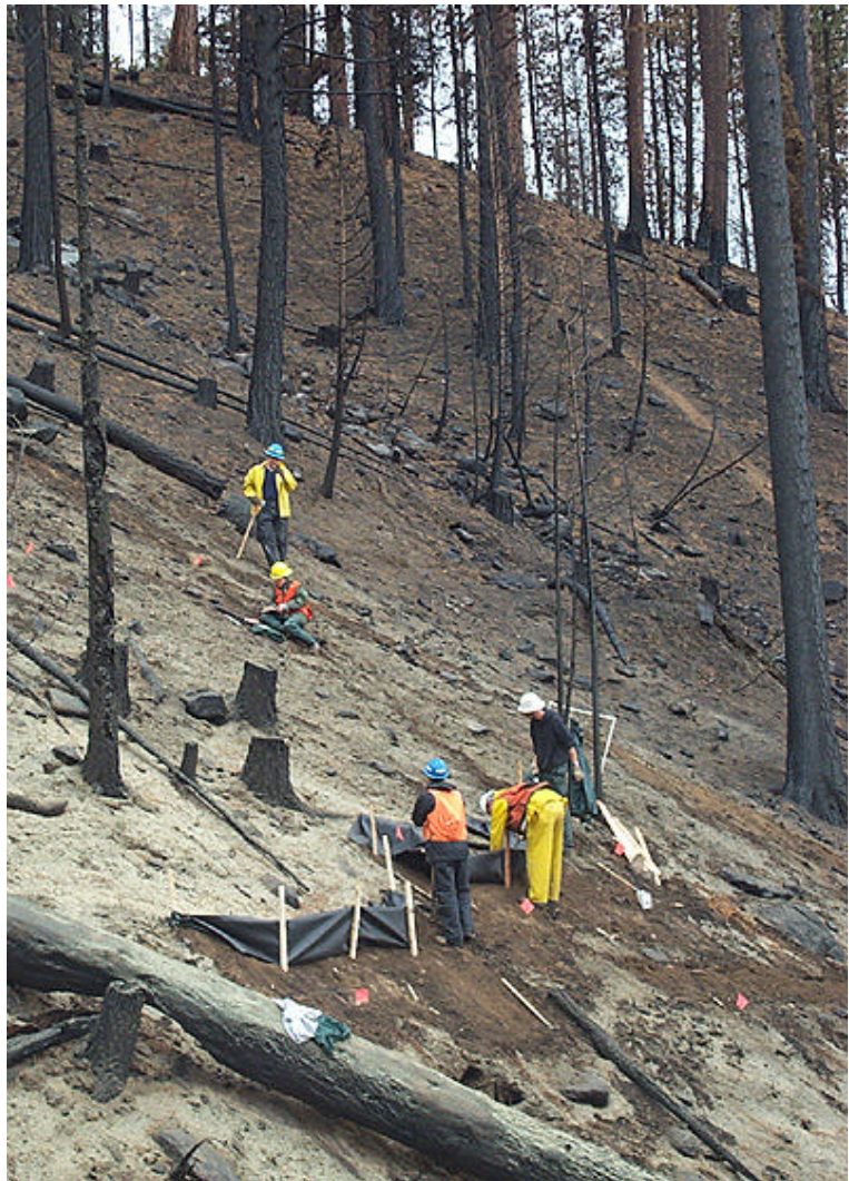
Installing silt fences to monitor the effectiveness of hydromulch after the 2003 Myrtle Creek fire, Idaho Panhandle National Forest.
